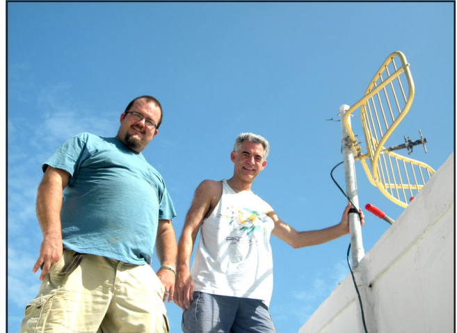
Improving the studio signal to Blue Mountain where WIVH's transmitter is located was accomplished by the installation of a larger microwave dish. Jonathan Bowman and Tim Madeira are pictured here.
